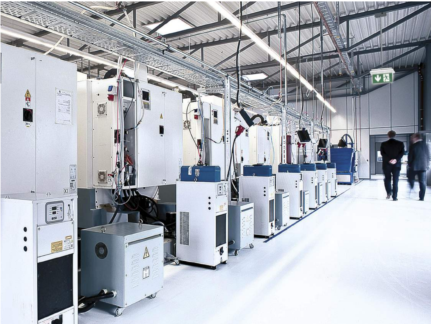
Industrial Area Emergency Lighting Application
