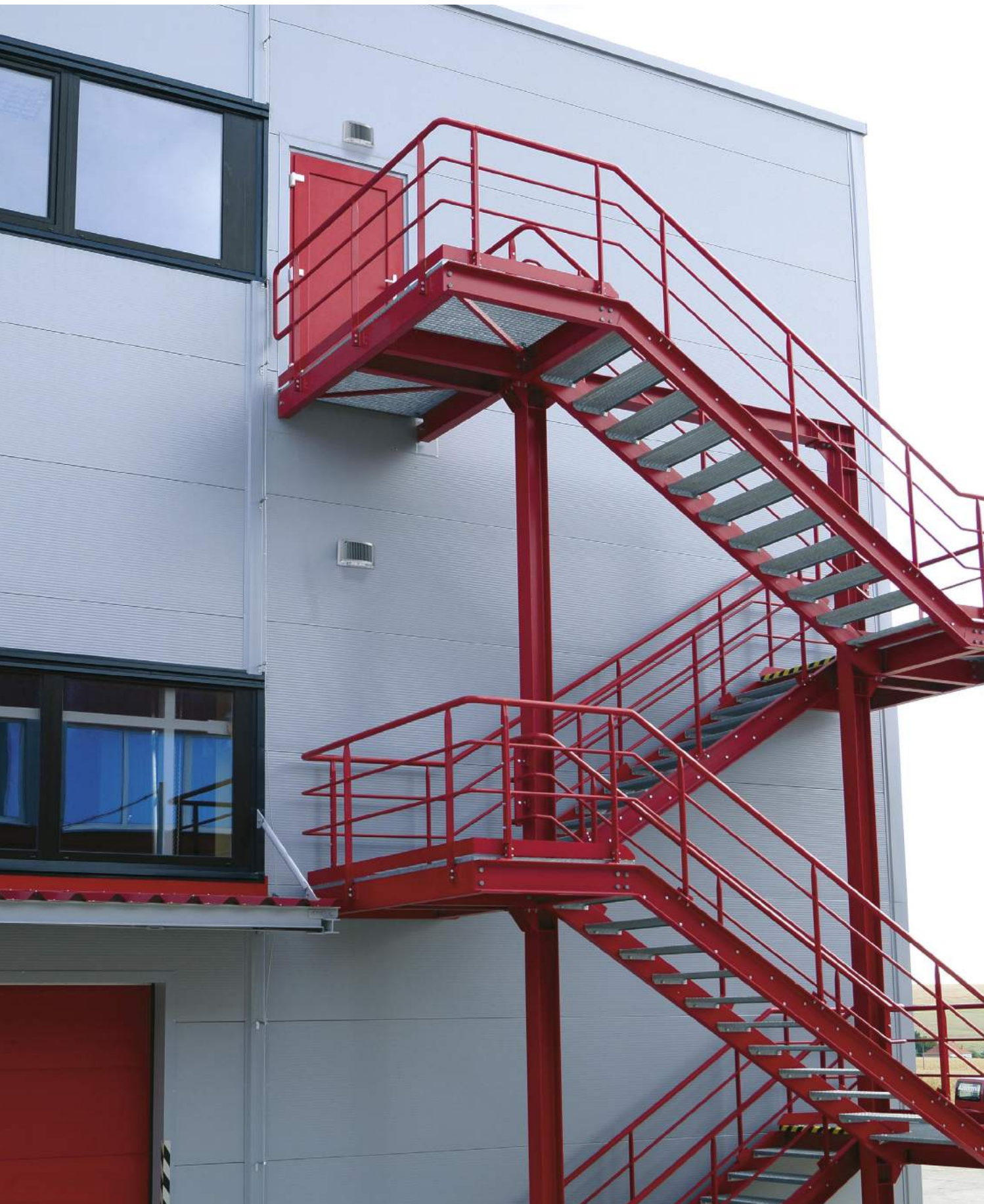
Outdoor stairs emergency lighting application
