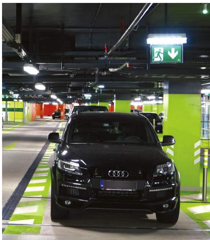
Parking Garage Area Emergency Lighting Application
