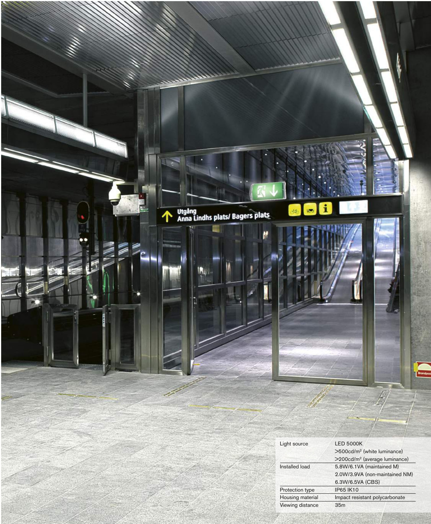
Train station area emergency lighting application
